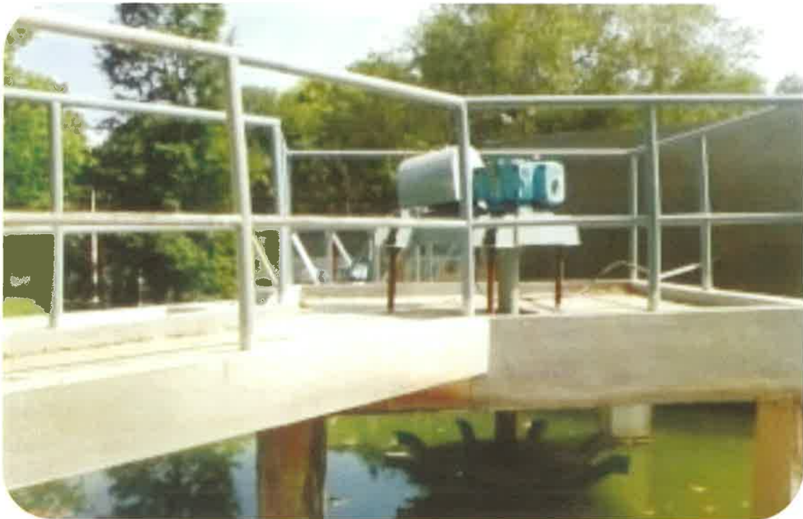
Sewage Treatment Plant, Madurai Prison
